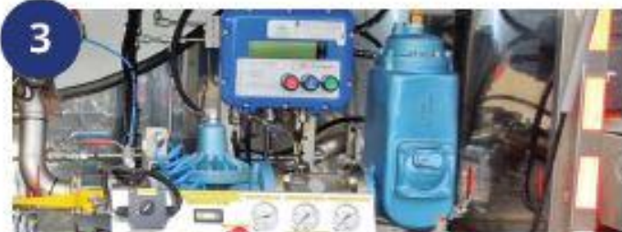
3 ALMA turbine flow metering system, popular in France.
