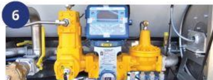
6 Combination of Liquid Controls mechanical flow meter MA-7 with S.A.M.P.I. electronic head, used mainly in Poland, Romania and Bulgaria.
